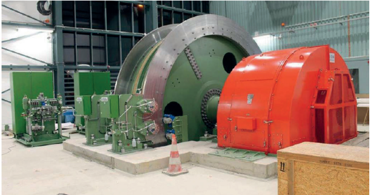
Fig. 4 Copyright 2022 BGE: Koepe winder North with drive. Image used with the kind permission of The Federal Company for Final Waste Disposal.
